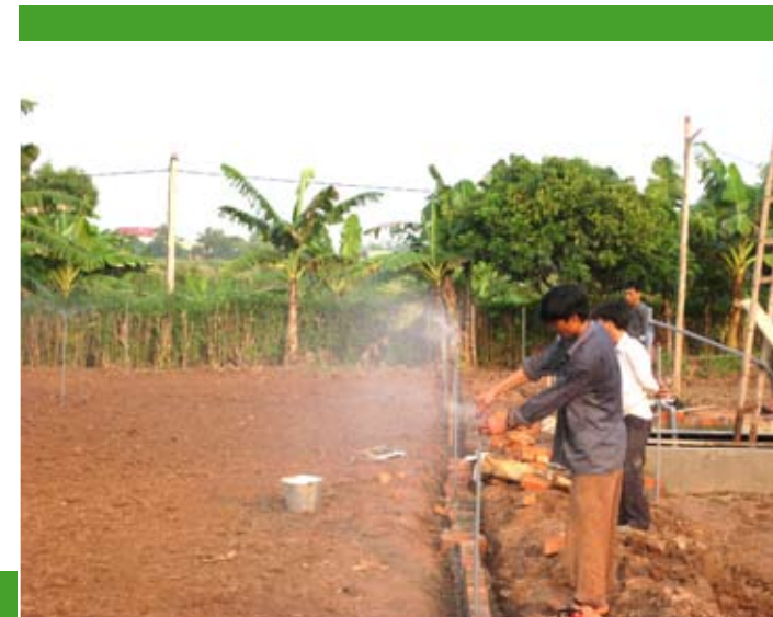
Sprinkler sticks with sprinkler and red deflector
